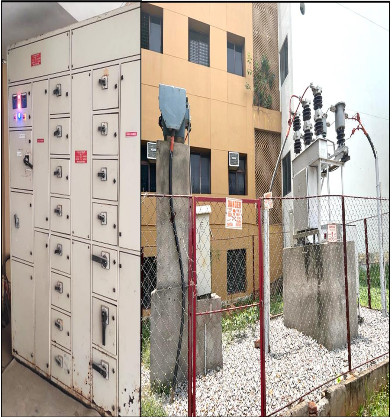
Power room and Transformer Facilities available in BIET Campus, Hyderabad
